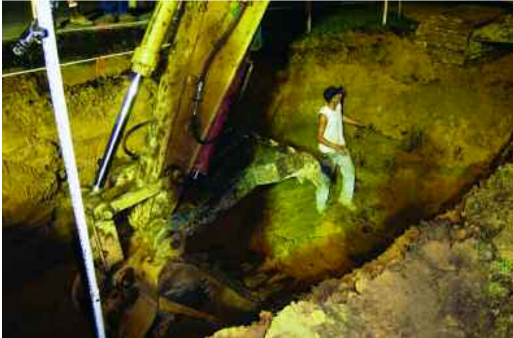
Figure 2: Monitoring of development projects, although often tedious and at odd hours, has yielded important information. In this photo, the hoe is excavating for a sewer along a public road to serve a new office building. The hoe has just uncovered the base of a brick foundation 10 feet below grade, where the man is standing. The profile along the road revealed two or three earlier roads, the first made with tar and chip around 1923, at more than 9 feet below the present surface.
